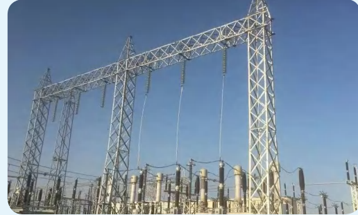
Djibouti Power Transmission and Distribution Project
