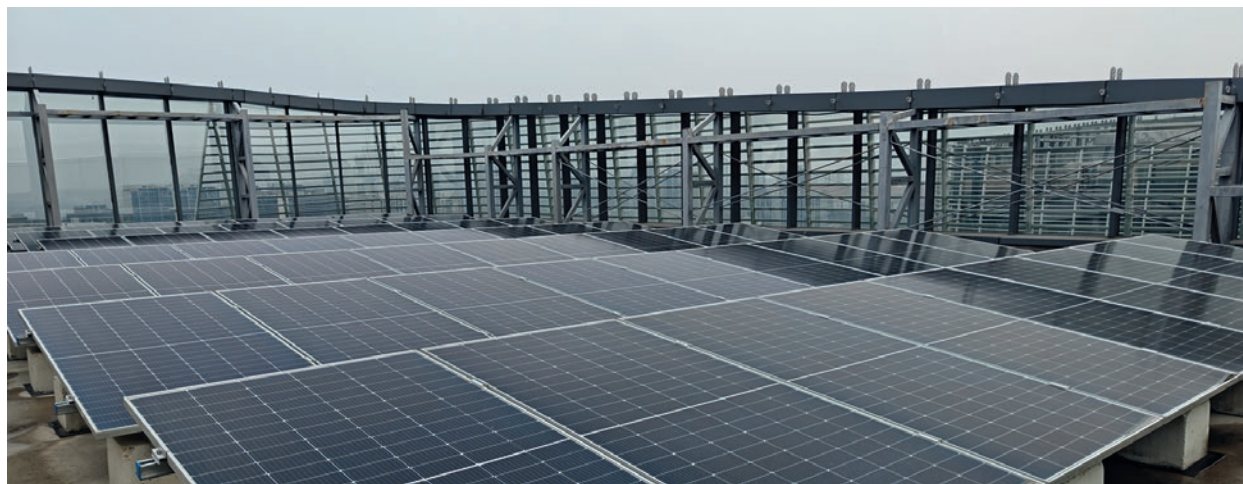
Photovoltaic Site Photo
