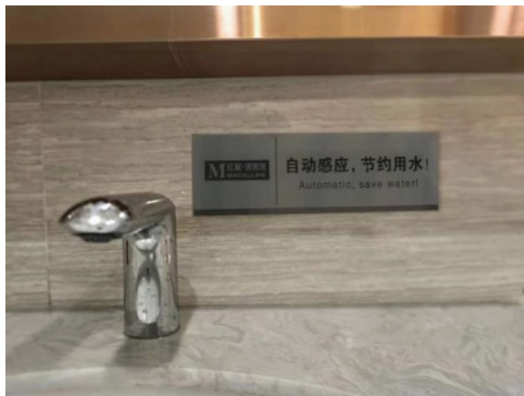
Sensor Faucets and Water Conservation Signage in Malls
