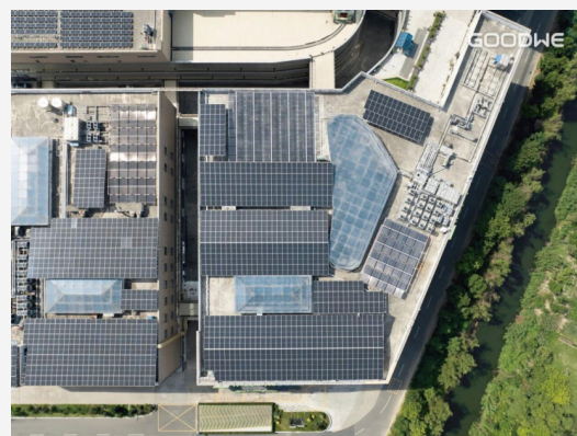
Nantong MACALLINE Rooftop Photovoltaic Project
