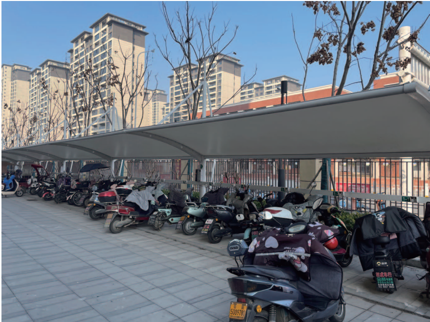
EV AC charging points located at The Xixian Kangqiao Xueyuan project
