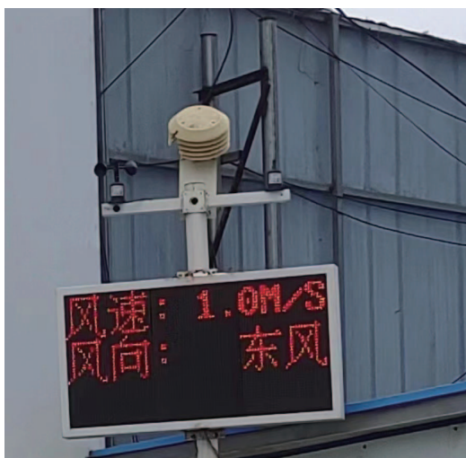
Air quality monitoring system installed on site
