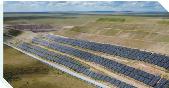
The Photovoltaic power generation system constructed by Breton
