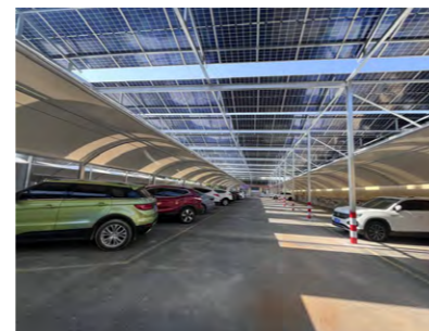
Linglong Gold Mine Photovoltaic Power Generation Device
