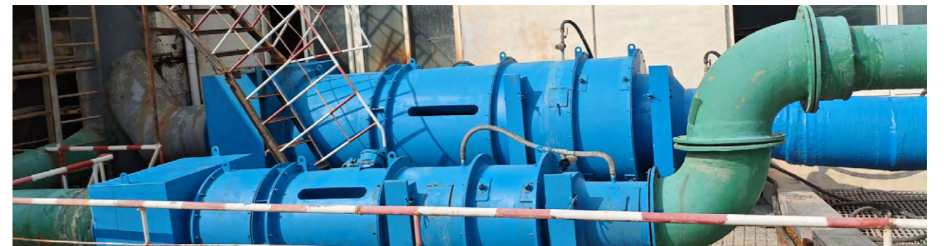
Xincheng Gold Mine Crushing Dust Removal System
