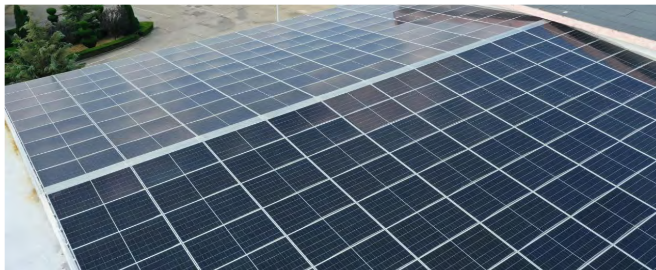
Gold Smelting Company Photovoltaic Greenhouse
