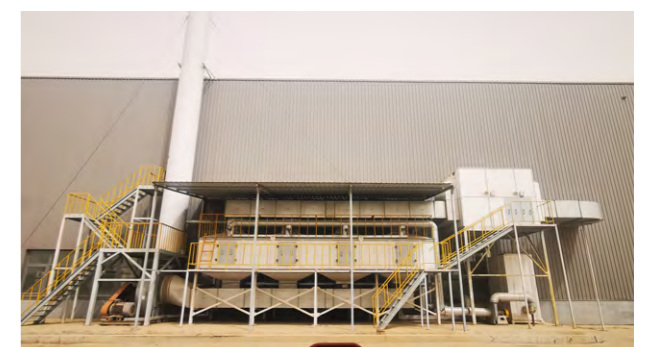
Paint Spray Exhaust Treatment Equipment
