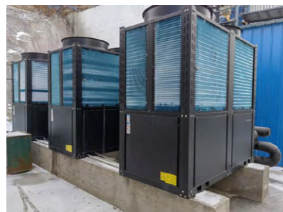
Shandong Jinzhou Group Air-source Heating
