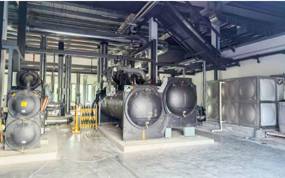
Laiwu Factory Ground Source Heat Pump System
