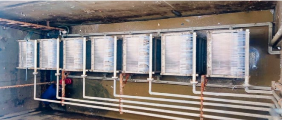
Update of the Biofilm System at the Wastewater Treatment Station
