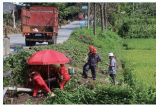
圖：合川公司錢塘鎮鄉村管線碰口作業 Picture: Hechuan Branch conducted rural pipeline tie-in work in Qiantang Town
