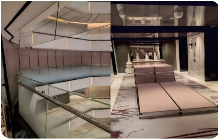
Picture: Enclosed hoardings and modular assembly to isolate noise, dust and odours, ensuring a healthy environment for guests
