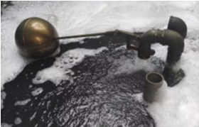
Automated Water Replenishment Achieved by Float Level Gauge
