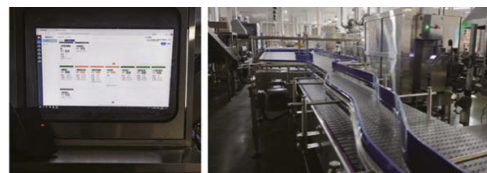
設備互聯與數據採集系統 Equipment Interconnection and Data Collection System
