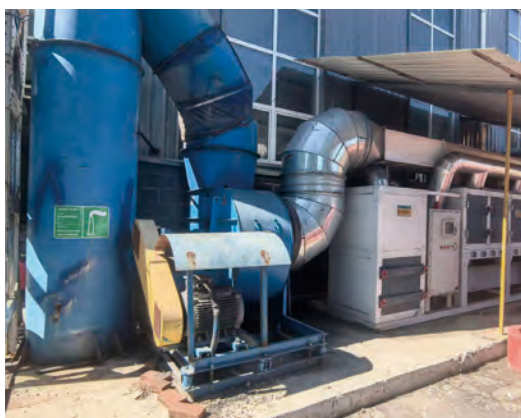
Exhaust air treatment equipment
