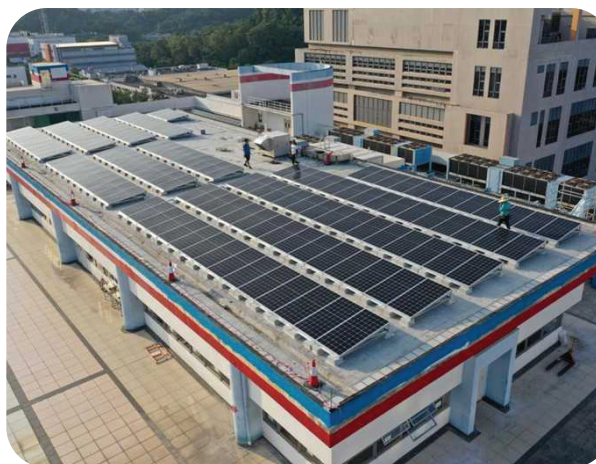
The 220-kW solar PV modules installed at the roof top of Lam Soon Building in Hong Kong
